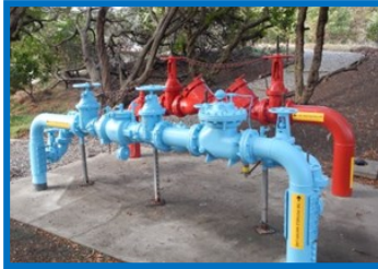
Potable (blue) and fire protection (red) water piping newly coated.
