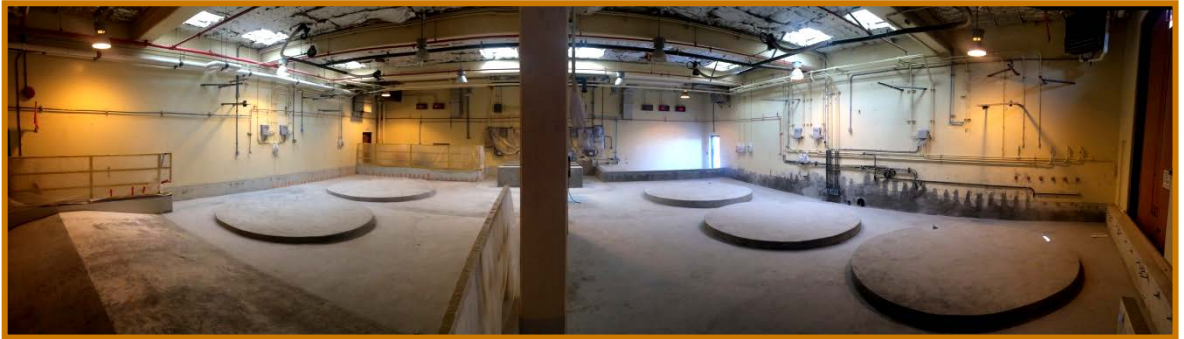
Interior of Chemical Storage Room, showing newly poured concrete floor and tank pads.
