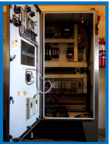
Inside the centrifuge control panel.
