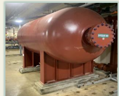
Recycled water tank
