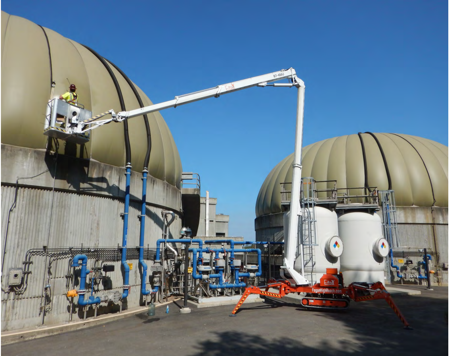
Contractor utilizing a “Spider Lift” to perform a membrane cover inspection on both anaerobic digesters.
